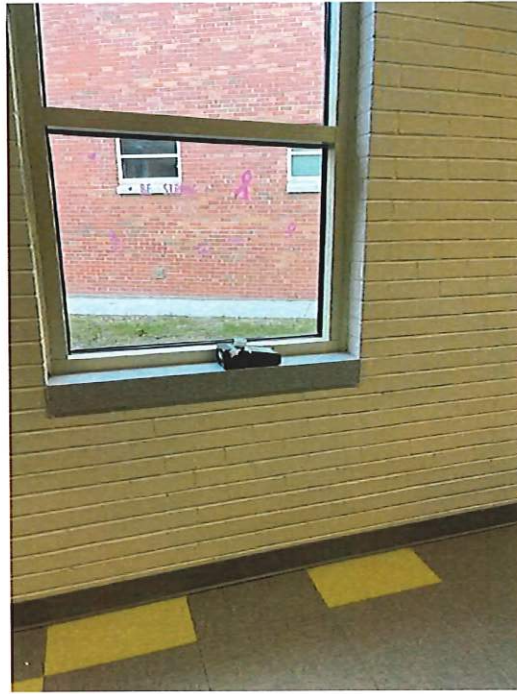
Figure 29. Green Wing Hallway and location of clearance sample A4. Figure from re-test taken on November 7, 2023.
